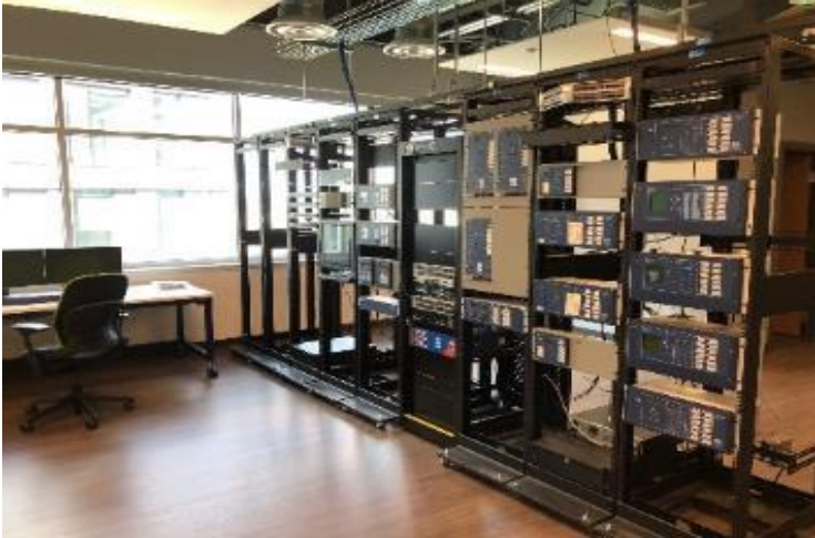
Power & Control Hardware in the Loop
